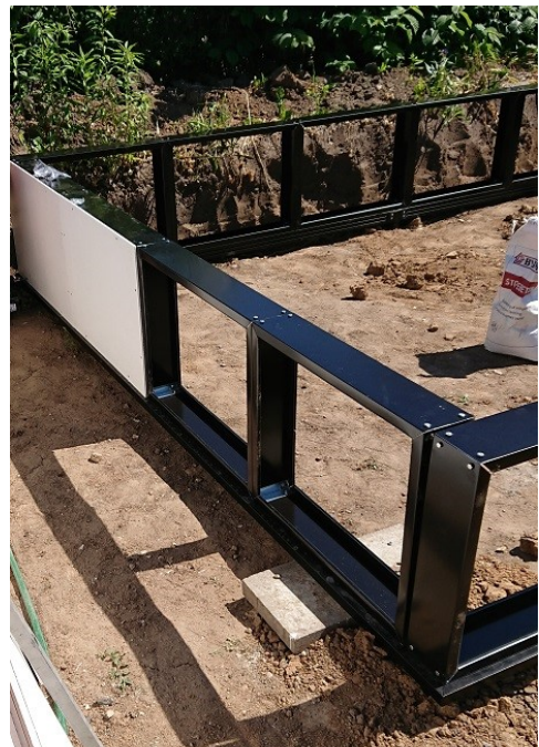
2) The profiles are then positioned on the perimeter foundation and the modular system is assembled from there.
