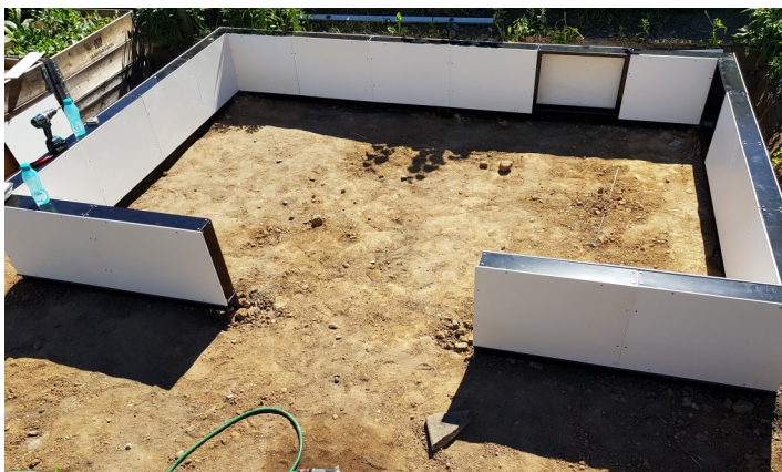
3) The cement fiber boards are attached with screws to the interior and exterior profile frames.
